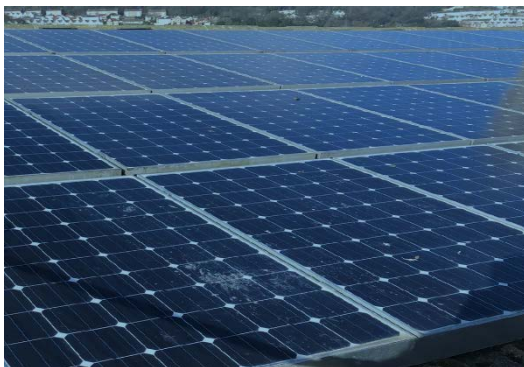
Solar PV modules installed on the Guildhall
