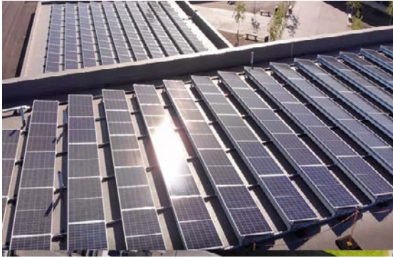
Solar PV on three comprehensive schools Pentrehafod, Gowerton and Pontardulais.
